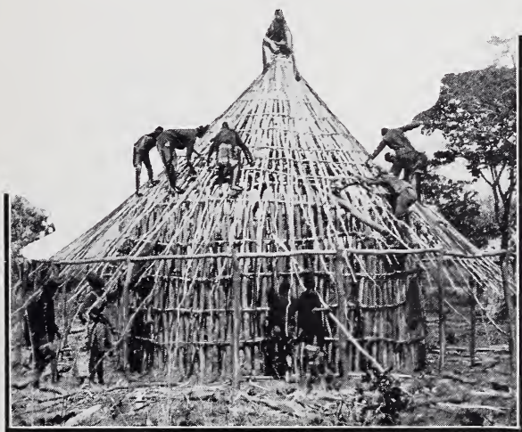
Angonis building a hut of poles. The sides will be plastered with clay and the roof thatched with grass. The men put up the poles and the women do the rest of the work.
